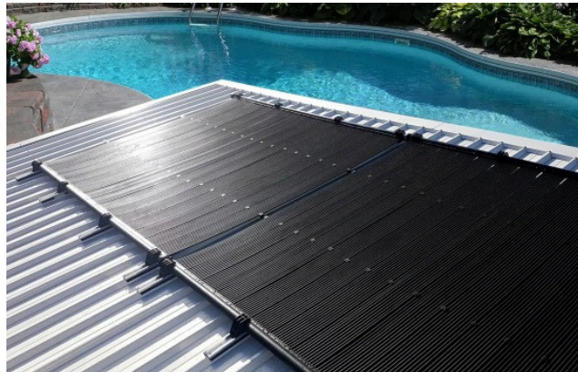
Solar Panel Pool Heating
